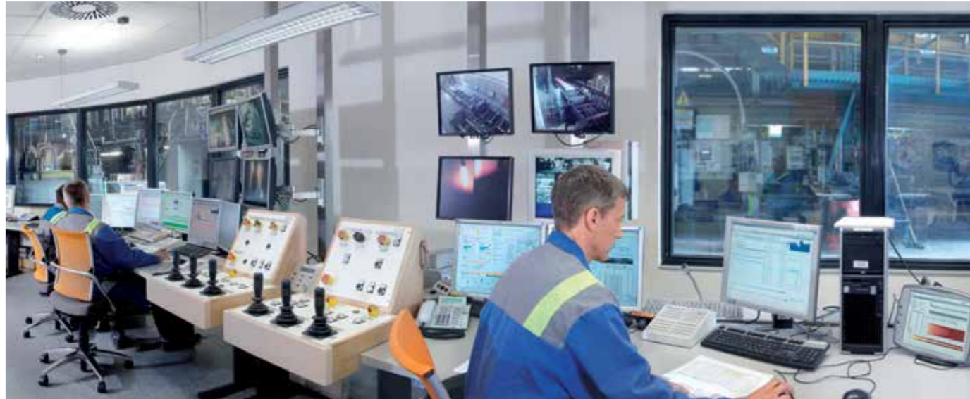
Continuous casting CC5 and CC6 control room, voestalpine Stahl GmbH, Linz, Austria
